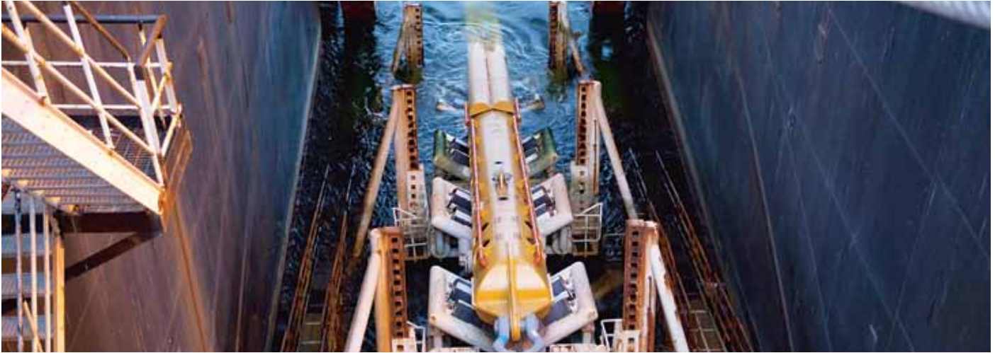
The last pipe of Line 2 laid by Allsea's Solitaire is lowered onto the seabed with the PIG (pipeline inspection gauge) launcher attached to it. The pipeline is built in three sections, which will be welded together only after they have passed pressure testing. This is expected to take place in the spring of 2012.
