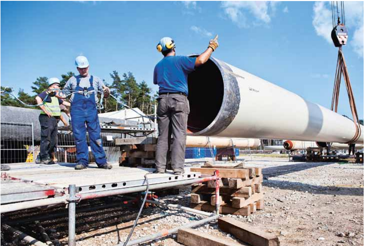
Lubmin: The 25-metre-long, 21 tonne, connecting segment between the onshore and offshore parts of Line 1 is positioned in order to complete the golden weld.
