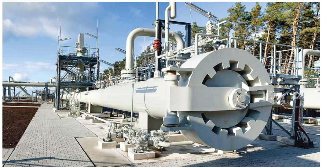
Above, a Pipeline Inspection Gauge (PIG) trap, houses the PIGs that have traveled through the pipeline from Russia.
