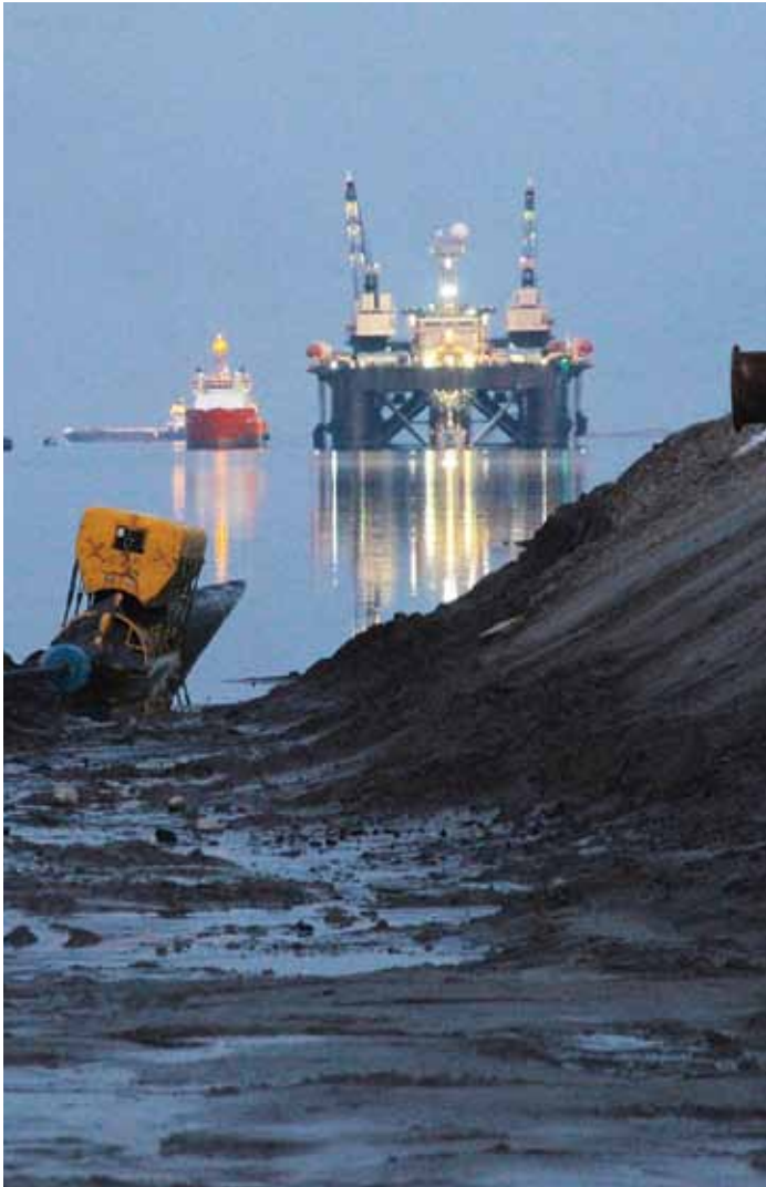
The first string of the pipeline was pulled onto Russian landfall on July 28, the second on August 4. The Castoro Sei is about 1,300 metres from the shoreline.
