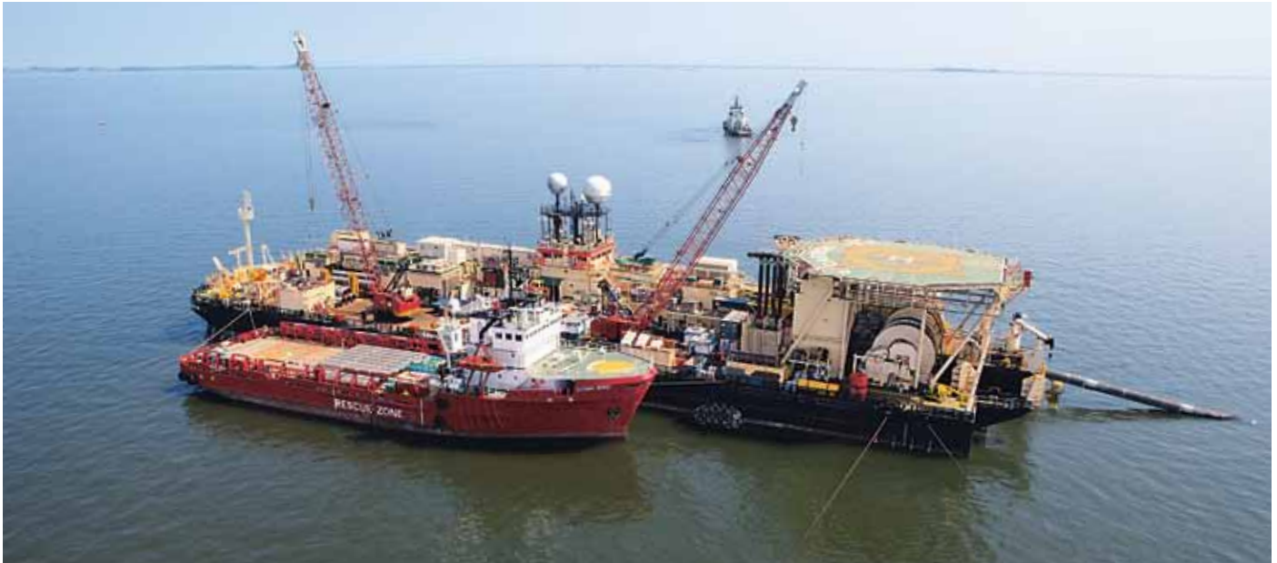
The Castoro Dieci, a flat-bottomed laybarge with low draught began working in the shallow waters of Germany's Greifswalder Bodden at the end of June. It is laying the shortest segment (28 kilometres) of each of the parallel pipelines.
