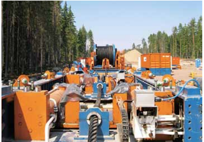
The pipelines were pulled ashore with the aid of a heavy-duty draw winch mounted on land. The winch weighs 100 tonnes.
