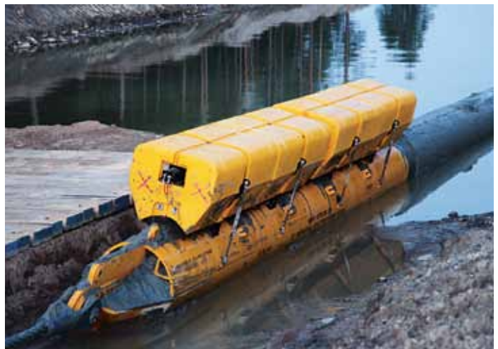
The tip of the pipeline is fitted with a pull head, to which a pull-in wire is attached. A buoy affixed to the pull head keeps it afloat as it is pulled ashore.
