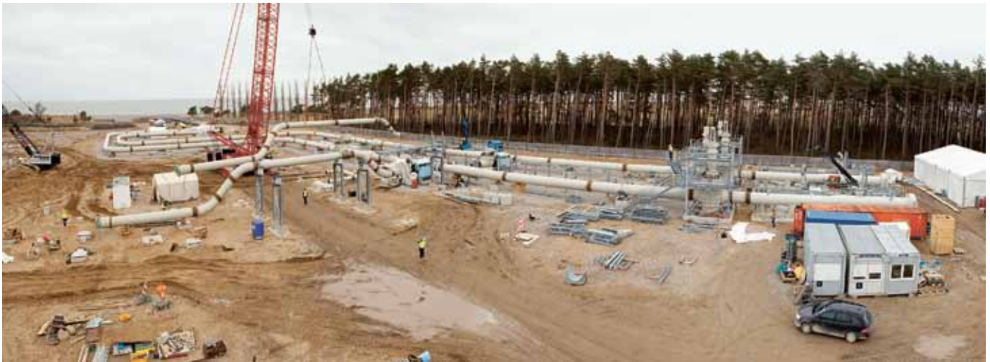
Offshore construction work involved in laying the gas pipelines at the German landfall was finished in December. Work is also progressing onshore.
