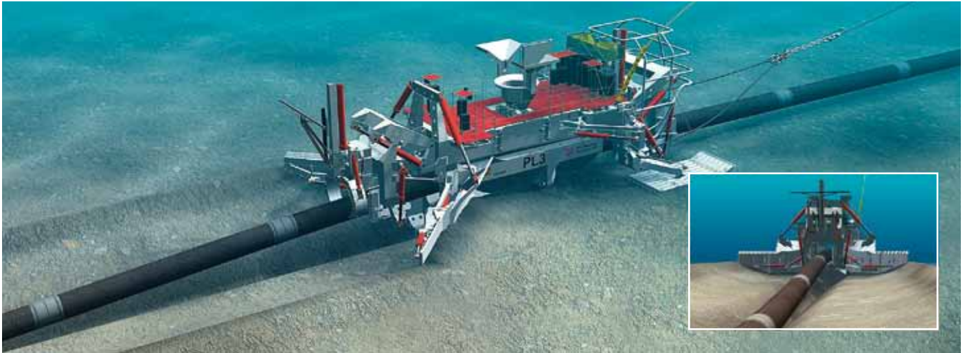
The PL3 raises the pipeline into its roller boxes, and is then towed by the Far Samson creating a trench into which the pipeline is laid as the plough moves forward.
